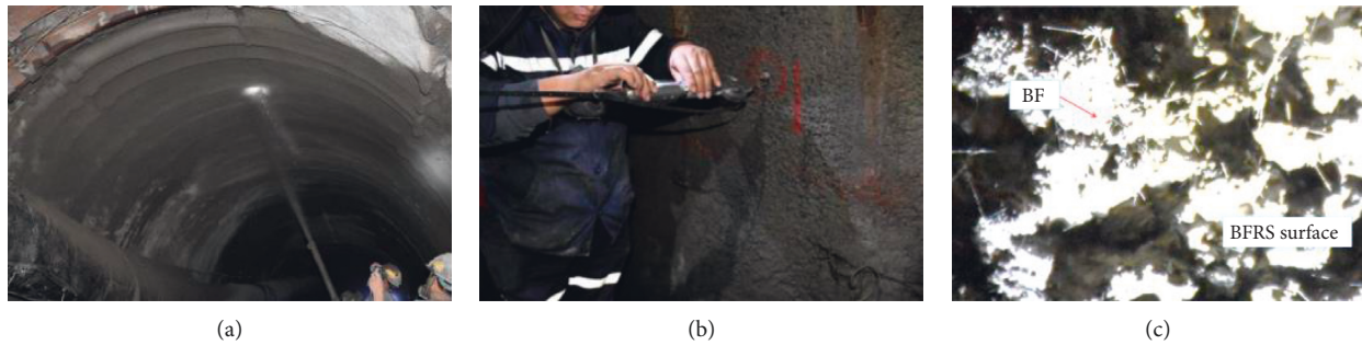
FIGURE 14: Shotcrete support of underground roadway: (a) concrete in-situ shot, (b) wall convergence monitoring, and (c) BF distribution on shotcrete surface.
