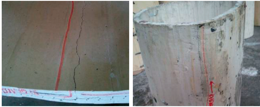
FIGURE 8: Lining cracks of reinforced concrete.
