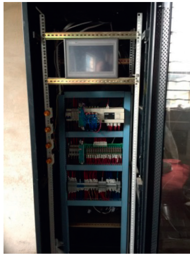
FIGURE 10: PLC data acquisition system.
