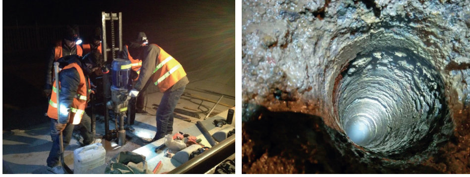
FIGURE 1: Fieldwork of the automatic monitoring system of moisture content of subgrade materials of high-speed railway in cold regions.
