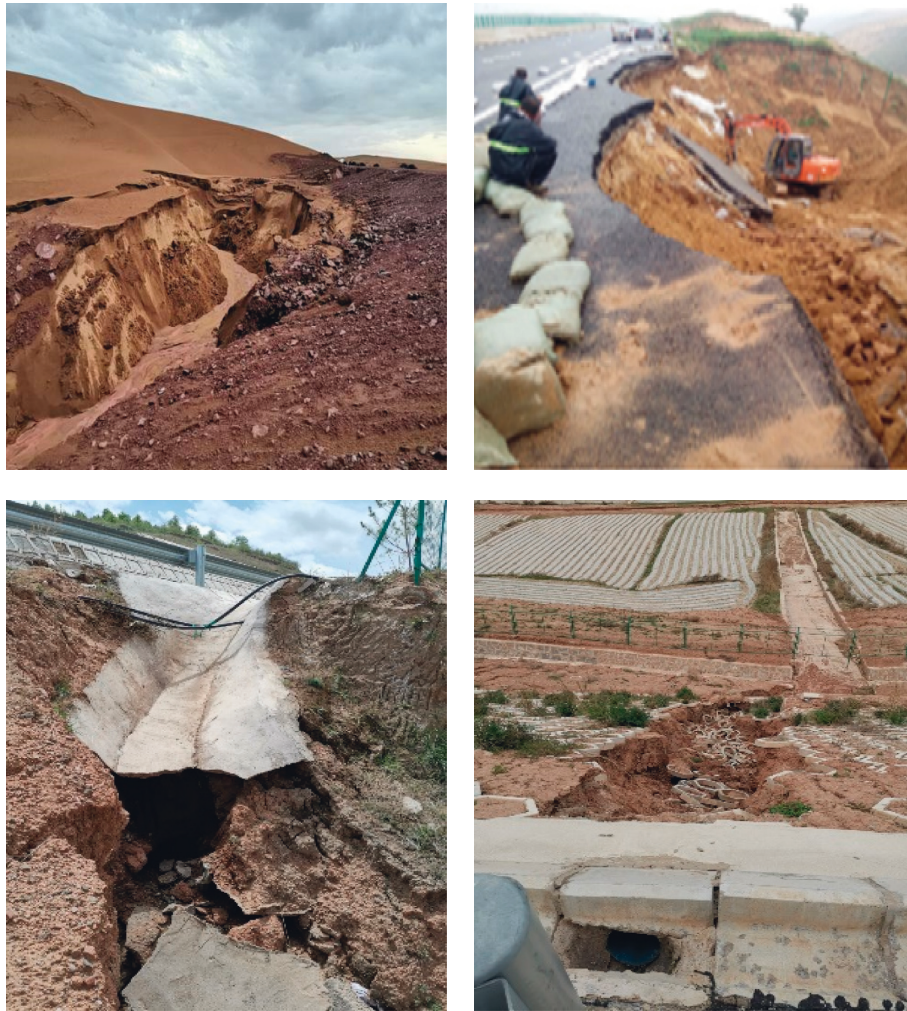
FIGURE 3: Picture of drainage ditch water damage site.
