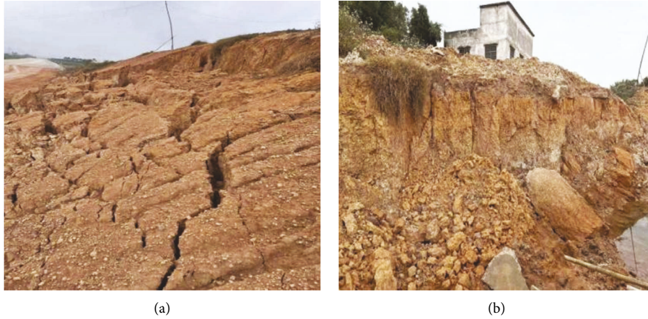
FIGURE 1: Cracking and collapse of expansive soil slopes.
