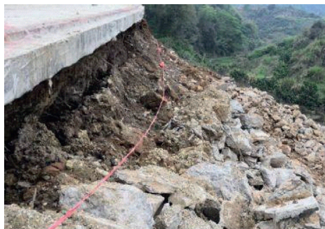
FIGURE 3: Actual pavement structure with voids.
