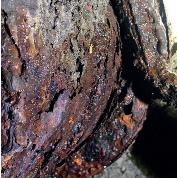
FIGURE 10: Severely rusted anchor head in the tailrace surge chamber.
