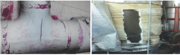
FIGURE 8: The damaged pneumatic pressure device.
