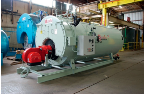
FIGURE 1: A power plant boiler in Iran.
