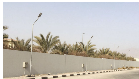
FIGURE 11: A section of the street where the luminaires are installed.
