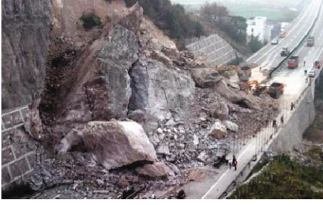
FIGURE 1: Collapsed highway slope.
