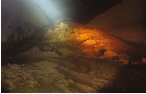
FIGURE 5: Gush of muddy fillings in F2 fault of Yonglian Tunnel.
