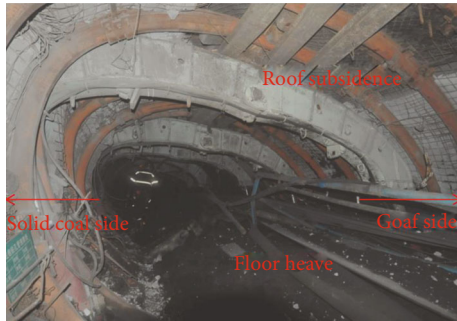
FIGURE 8: Main roadway destruction site.
