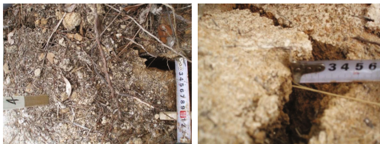
FIGURE 9: Fresh crack appeared in the monitoring range.
