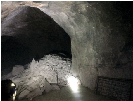
FIGURE 2: Rockburst at the intersection between lower drainage corridor and tailrace branch tunnel no. 1.
