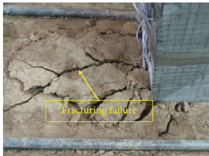
FIGURE 19: Fracturing damage of soil in front of pile.
