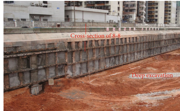
FIGURE 1: Construction photo of the pile-anchor structure at the west side of excavations.
