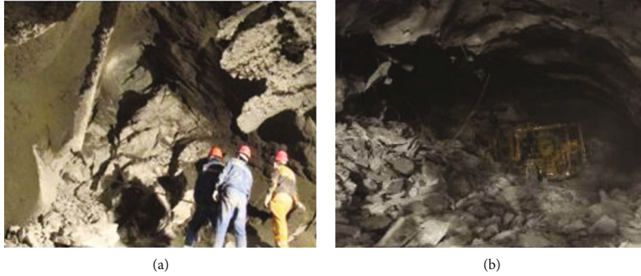
FIGURE 1: Excavation damage of Jinping tunnel. (a) Rock burst of Jinping tunnel on 28 November 2009 [6]. (b) Collapse of Jinping No. 4 drainage tunnel [7].
