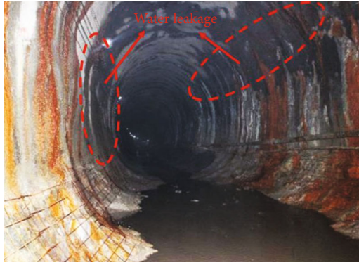
FIGURE 1: Water leakage in the subway tunnel.
