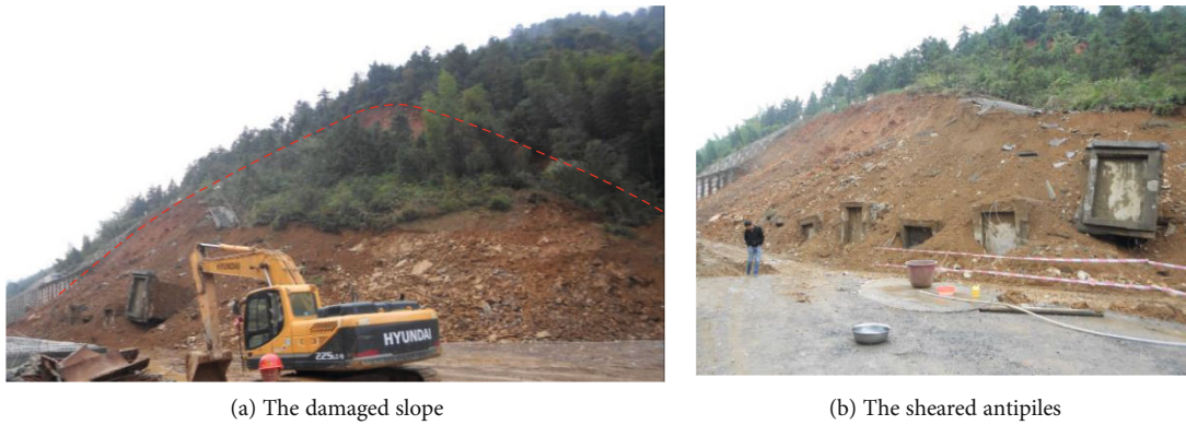
FIGURE 5: Photos of the landslide failure.
