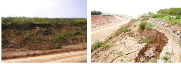
FIGURE 2: Collapse of expansive soil slopes.
