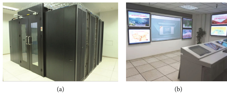
FIGURE 10: Tunnel intelligent remote monitoring data center management system and release system.
