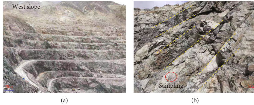
FIGURE 1: Rock mass structure of the Beizhan open pit slope, a set of dominant structural plane can be observed as drawn in orange color.
