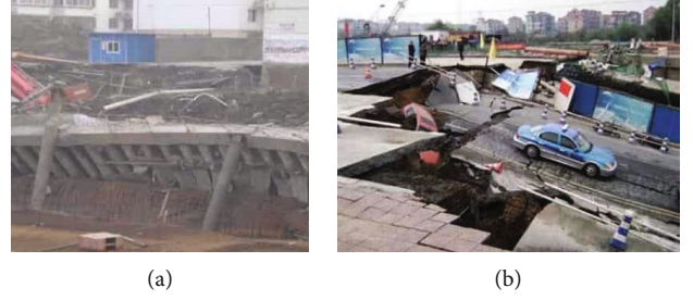
FIGURE 1: Typical foundation pit excavation accidents. (a) Foundation pit collapse accident in Suzhou in 2008. (b) Foundation pit collapse accident in Hangzhou in 2008.
