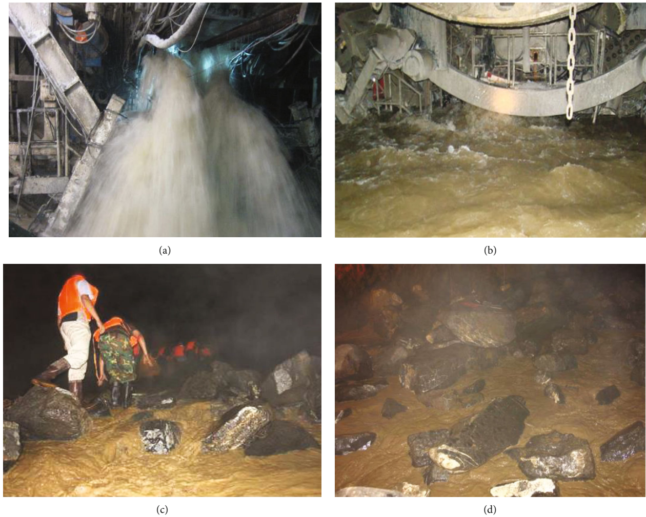
FIGURE 1: Typical geological disasters of water burst in underground engineering.
