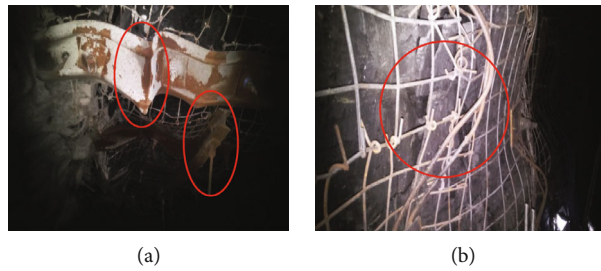
FIGURE 3: The failure of bolt-cable-mesh support: (a) steel belt bending and shear of anchor cable. (a) Failure of anchor net.
