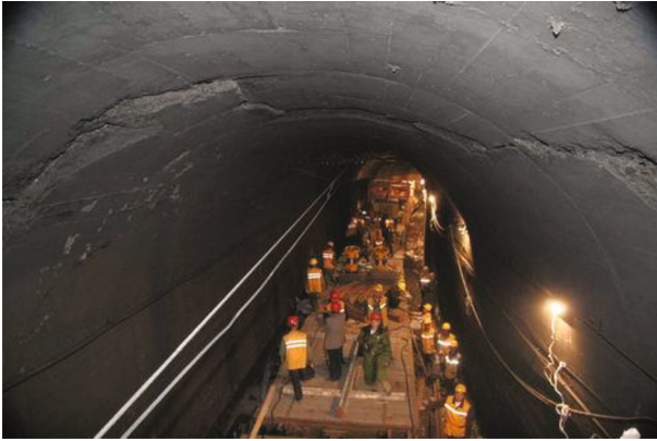
FIGURE 1: Cracking of tunnel lining.
