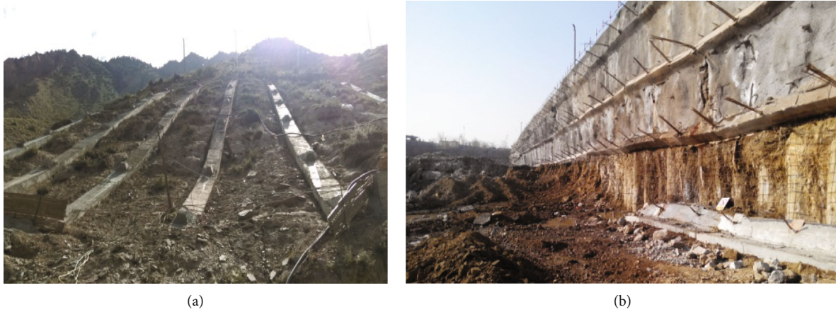
FIGURE 1: Application of prestressed anchor cable: (a) used in a high slope and (b) used in a deep foundation pit.
