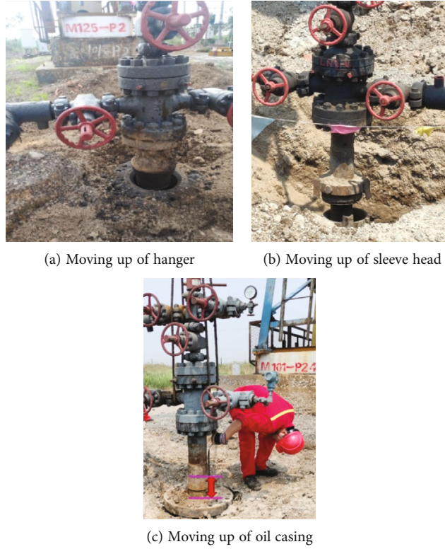
FIGURE 1: Damage mode of Jidong oilfield casing moving up.
