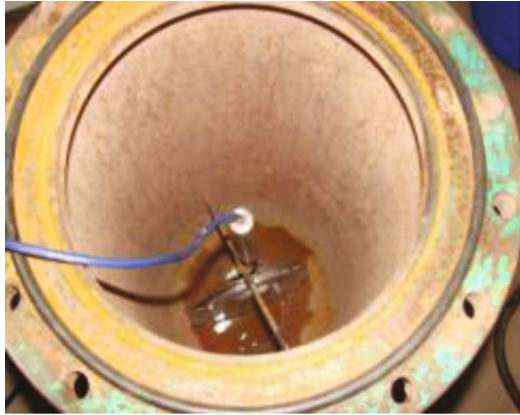
FIGURE 3: Installment of the pressure gauge in the pressure tank.
