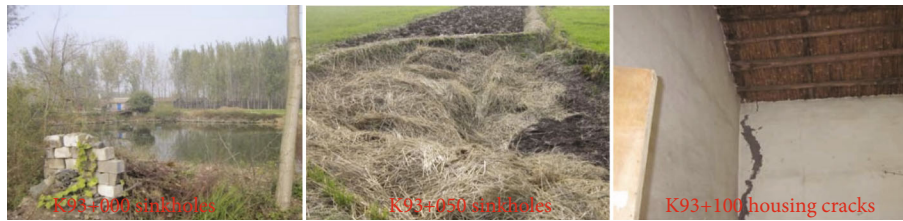
FIGURE 11: Ground collapse caused by goaf.
