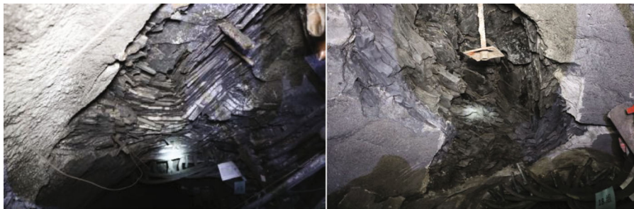
FIGURE 2: Bending deformation of roadway roof.
