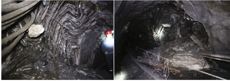
FIGURE 3: Rib deformation of roadway.
