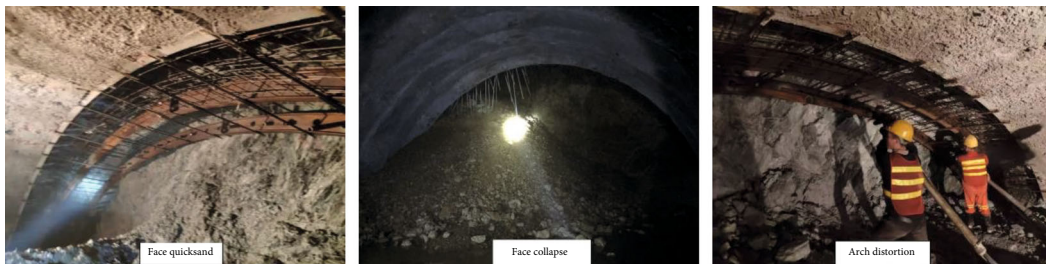
FIGURE 1: Tunnel face accident.
