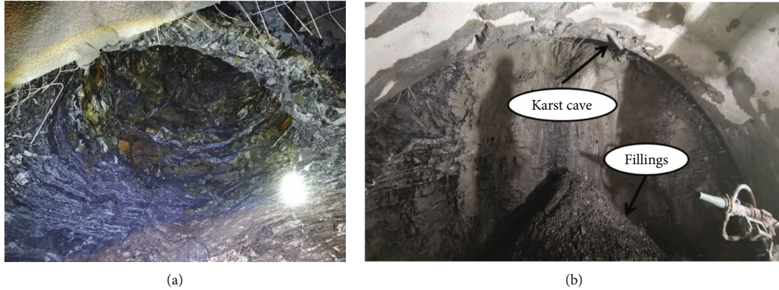
FIGURE 1: The condition of the palm surface at DK114+070: (a) karst cave and (b) fillings from the karst cave.
