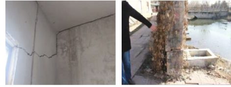
FIGURE 1: Crack and dislocation of fixed brick-concrete structure pump house under coal mining subsidence.
