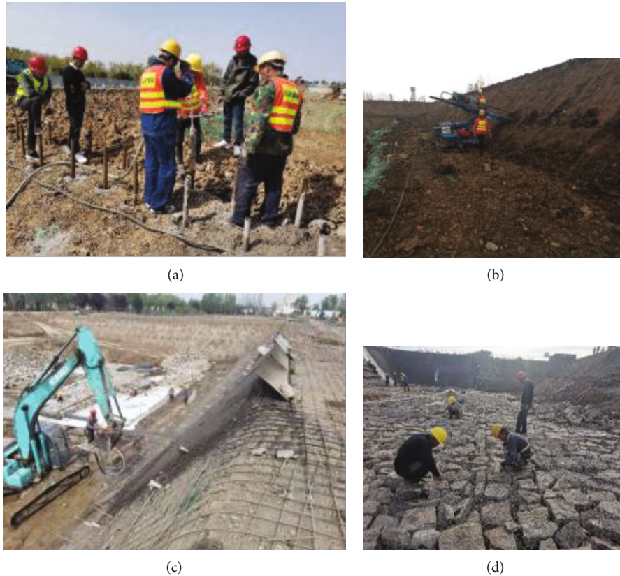
FIGURE 10: Site construction of boat pond reinforcement: (a) curtain grouting; (b) excavation and backfilling of foundation pit; (c) slope support; (d) boat pond construction.
