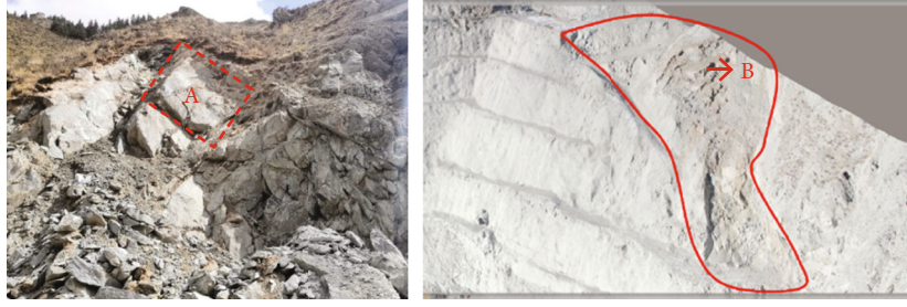
FIGURE 4: Sliding-slip perilous rock on both banks of the dam site.
