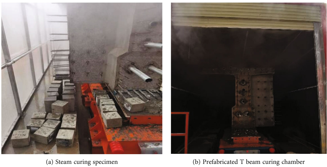
FIGURE 2: Steam curing chamber.
