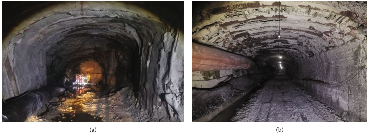
FIGURE 15: Comparison of roadway stability before and after pressure relief: (a) before roadway pressure relief; (b) after roadway pressure relief.
