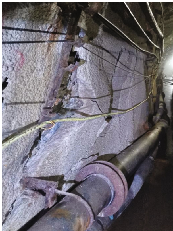
FIGURE 1: High-stress-induced instability of surrounding rock.
