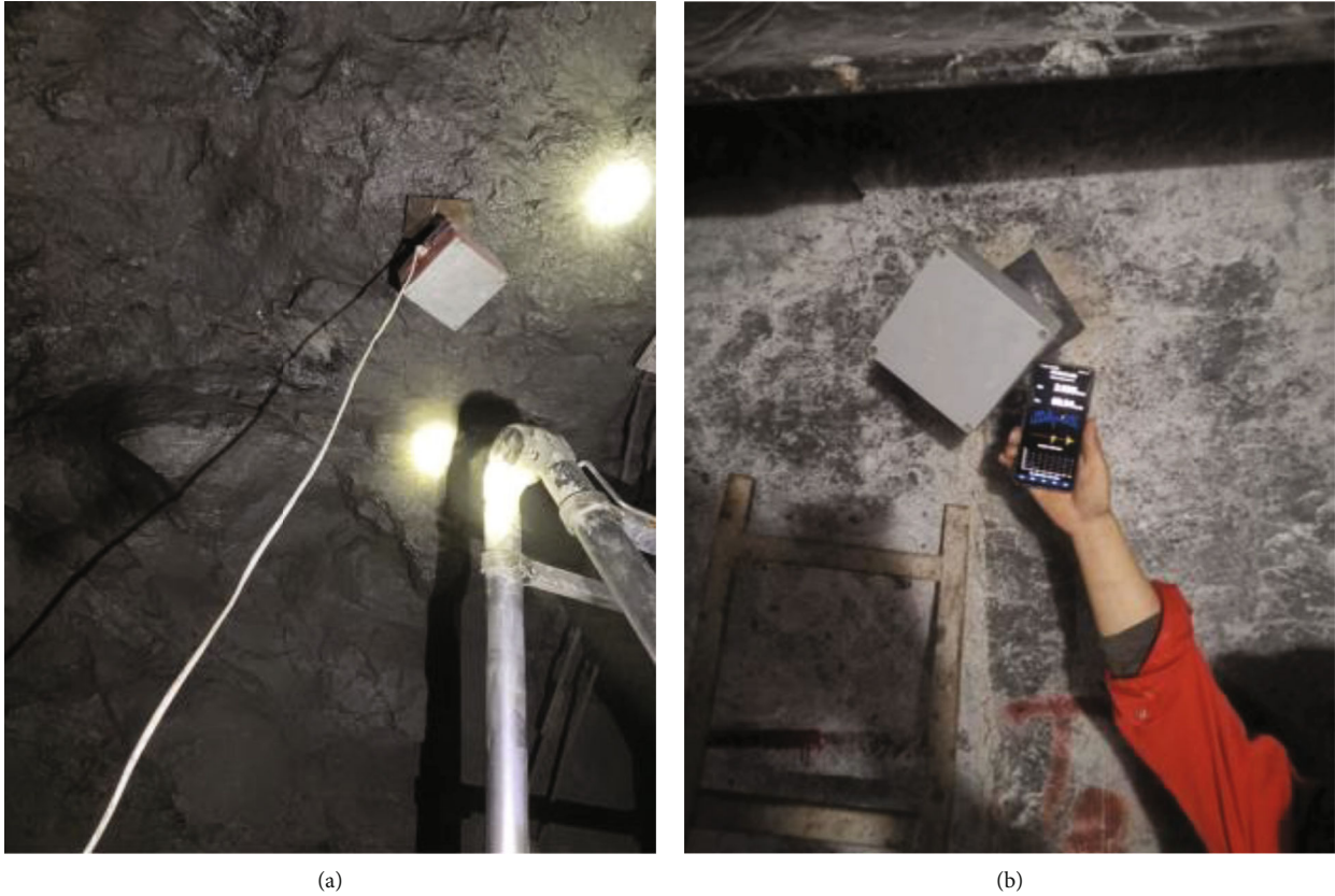
FIGURE 17: Installation position of system: (a) location of pressure relief roadway; (b) location of main roadway location.
