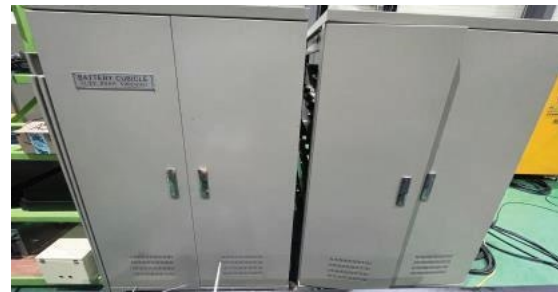
Battery 56 kWh, 1.2V 80 AH 590 cells
