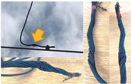
FIGURE 46: Caged jumper near overhead line neutral section.
