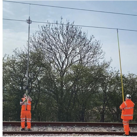
FIGURE 49: Staff installing a rigid stainless steel dropper on the ground that the left staff is installing while the right staff is pushing up the wire.
