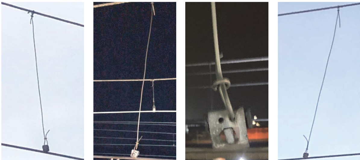
FIGURE 15: Droppers coming off contact wire.
