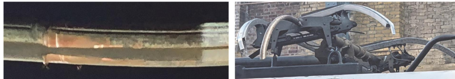
The dragging mark on the contenary wire
