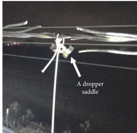
FIGURE 28: Dropper's top loop cuts into aluminium–steel catenary wire.
