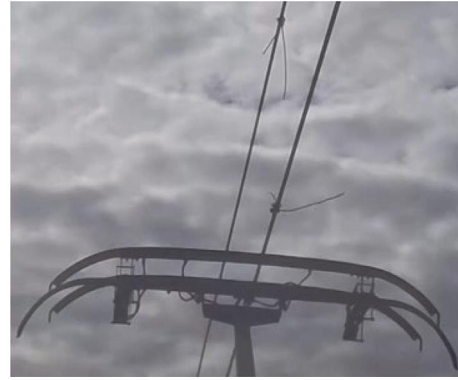
FIGURE 1: Broken dropper wire that could affect pantograph operation.
