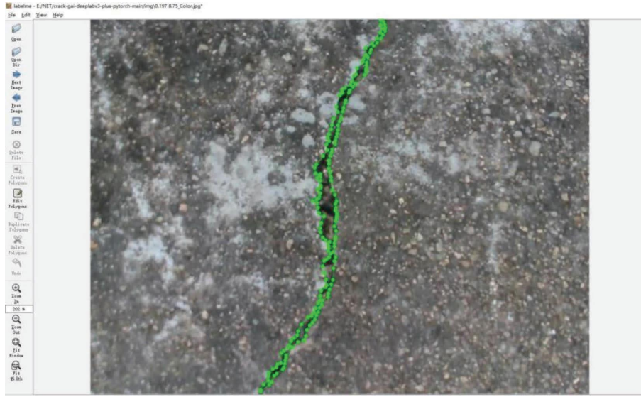
FIGURE 13: Labeling of the crack data with LabelMe.
