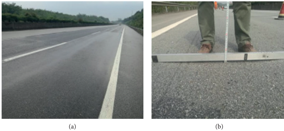
FIGURE 7: Rutting of Guangyun Expressway.
