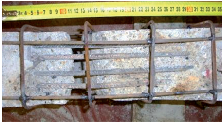
FIGURE 3: Typical installation of the jacketing steel reinforcement (view from the bottom of the original damaged beam).
