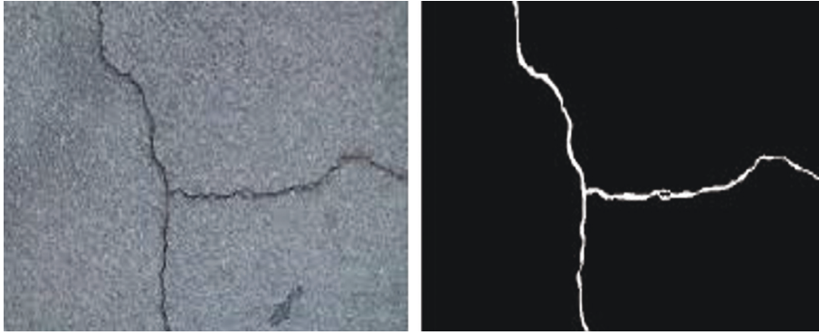
FIGURE 10: Deep learning-based crack segmentation [56].
