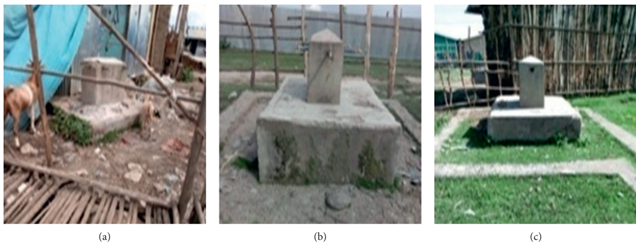
FIGURE 4: Nonfunctional public pipes (a–c) in the study area (photo by Girma Deboch, 2018).
