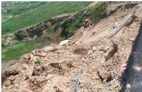
FIGURE 3: The trailing edge of the top of the landslide.
