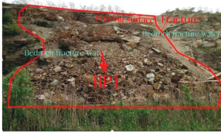
FIGURE 2: Scene of landslide 1.
