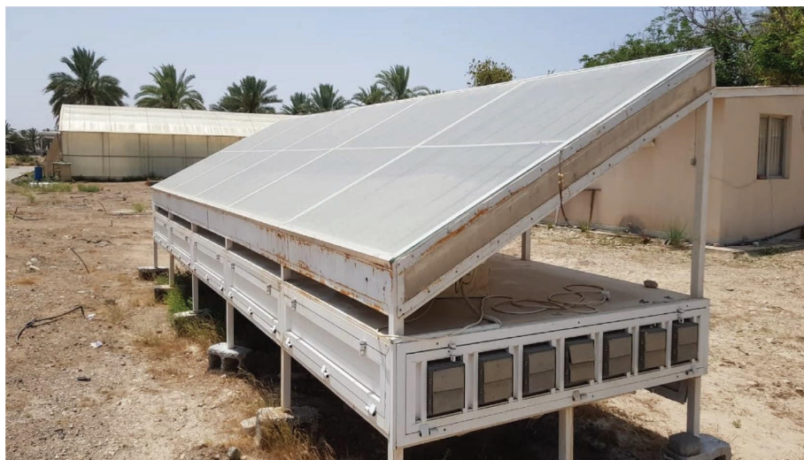
FIGURE 2: Installed forced convective solar dryer (FCD) at agricultural experimental station, SQU.
