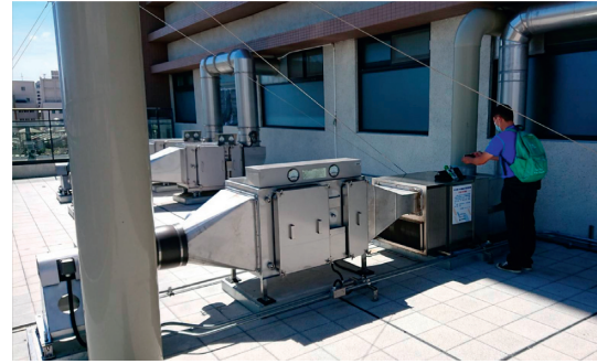
FIGURE 12: Picture of the completed full-outer-air-intake natural air-conditioning system for negative pressure isolation wards.
