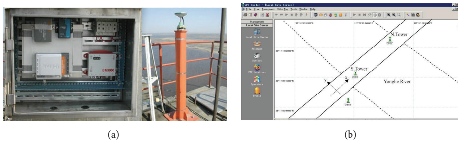
FIGURE 2: (a) Tower-GPS monitoring and (b) axes definition of the local coordinate system and locations of the GPS monitoring systems.
